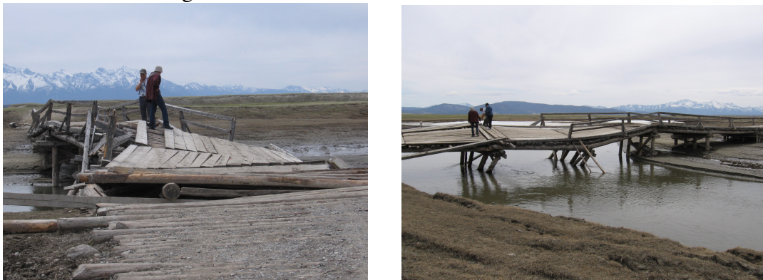
Figure 6. Examples of bridge failure, photograph courtesy of C. Montagne.
